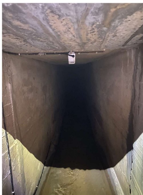
Sensor montert i taket
