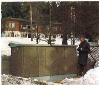
Transformer kiosk or substation.
